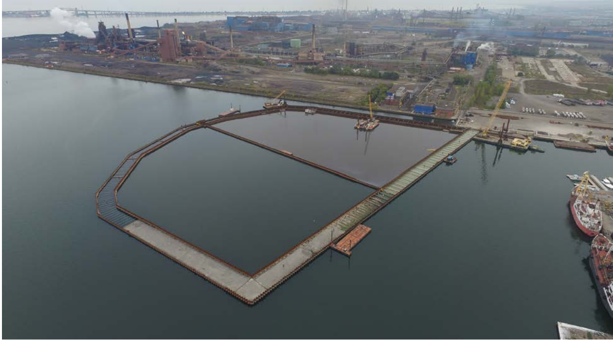
Construction of an engineered containment facility for contaminated sediment in Randle Reef, Hamilton Harbour. Credit: Hyperactive Productions.
