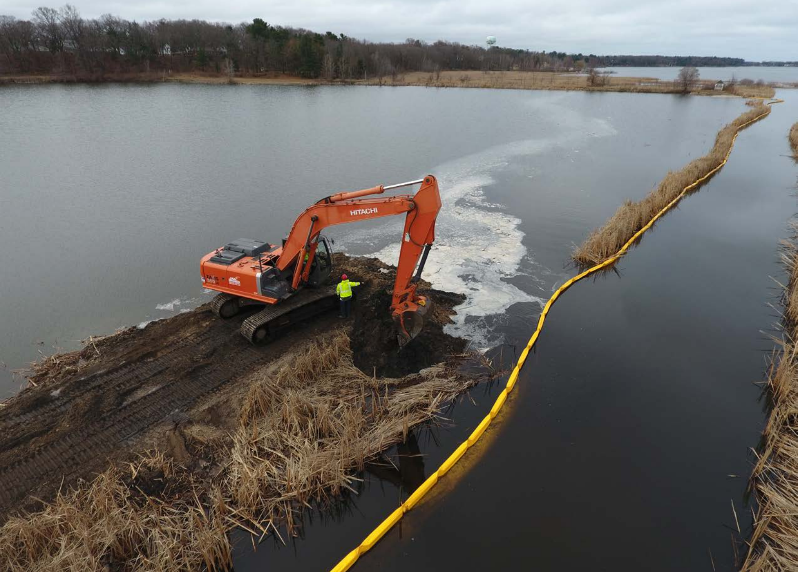
Berm removal to restore hydrological connection to Bear Lake. Credit: GEI Consultants of Michigan.
