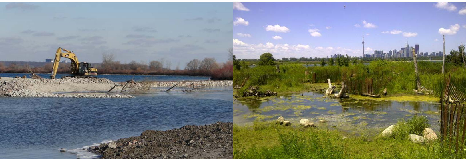
Construction of wetland at Embayment D, Tommy Thompson Park (left), and view of downtown Toronto through constructed habitat at Tommy Thompson Park (right). Credit: Toronto and Region Conservation Authority.
